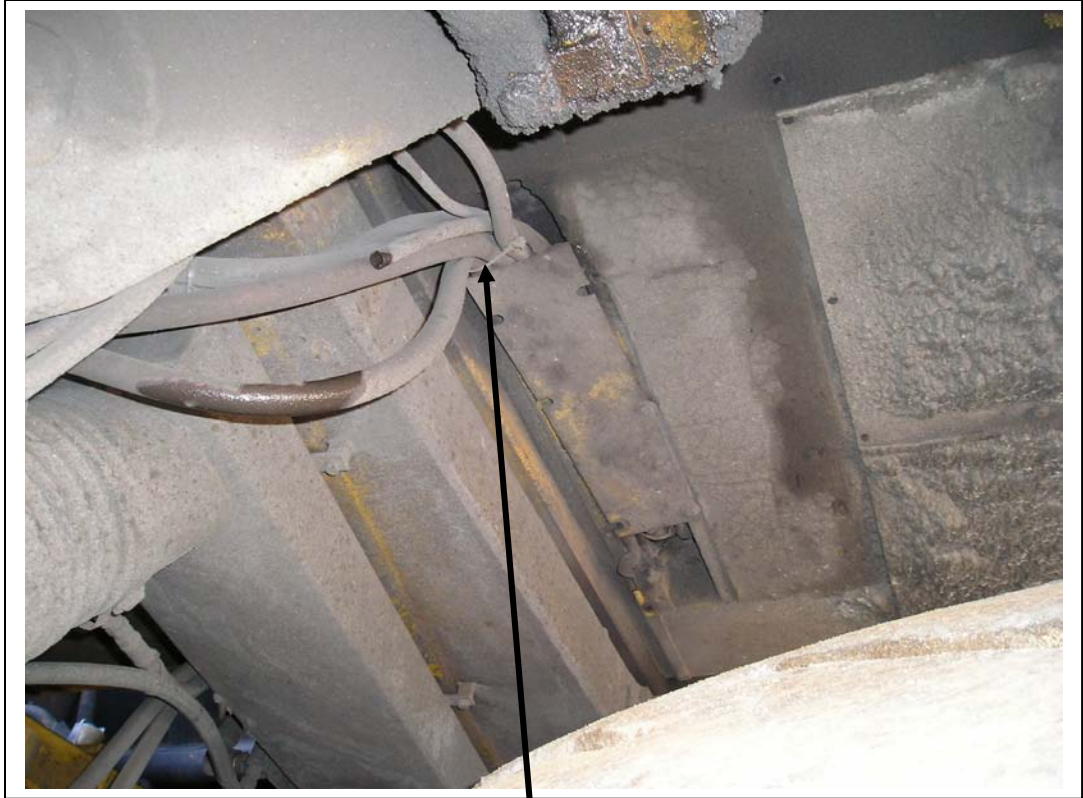
Hoses running out under the cab and down towards the engine.
